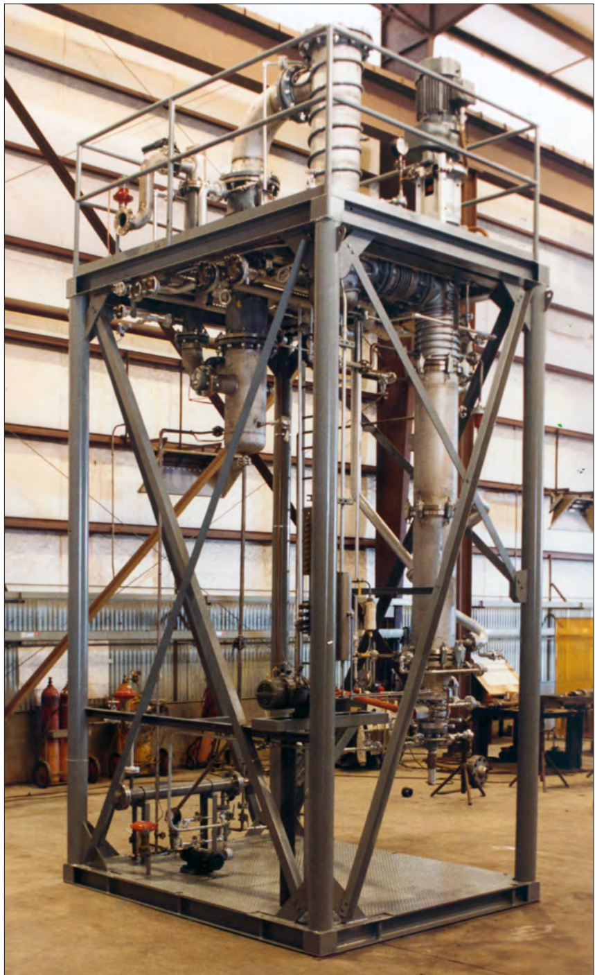
LCI skid mounted solvent recovery system
