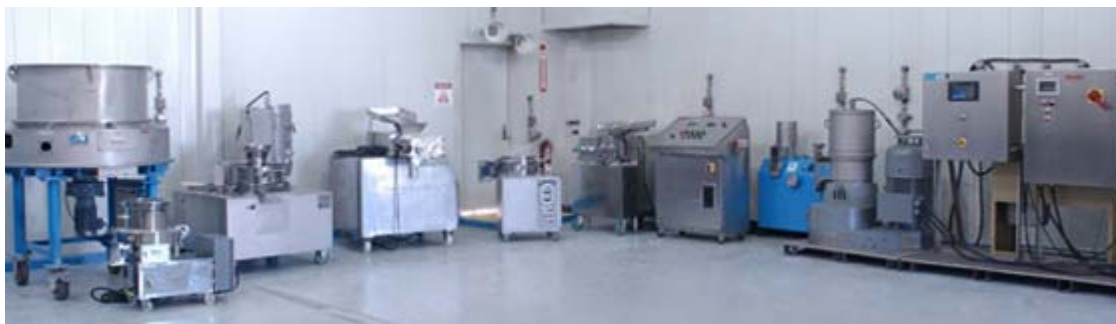
LCI's Pilot Plant
